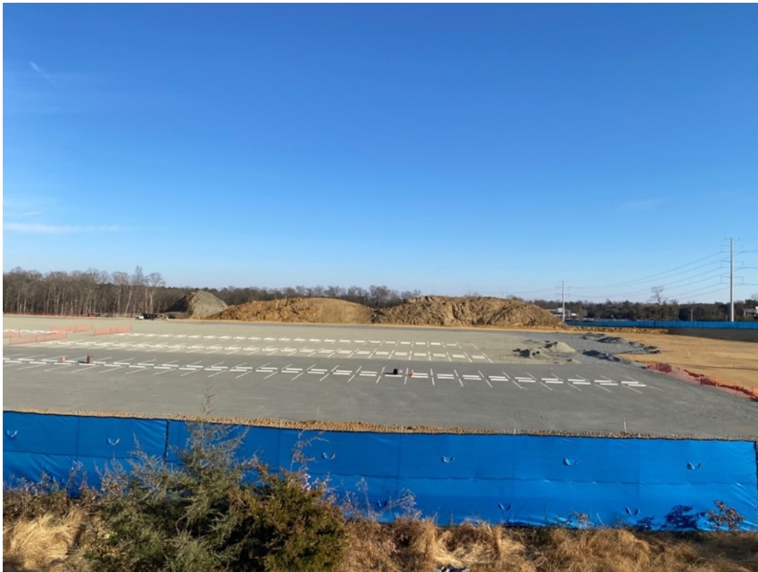
Figure 27. Data Center Development under construction near Manassas Battlefield and Pageland Lane on University Blvd. Note the flattening of topography and large swaths of pavement needed for this development typology. This aesthetic would replace the current rural aesthetic of the areas that the Thornton Drive Settlement and Marble Hill / Flat Iron Corner currently still have.
